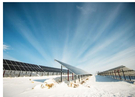
SOLAR POWER PLANT AT SVETLOYE
